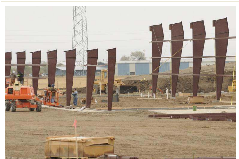
Williston Herald Contractors work on the new Williston Frontier Equipment Case IH dealership building last week as the steel frame is quickly going up.
